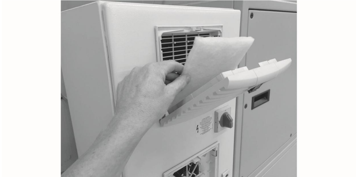
Fig. 57: Filter replacement in control cabinet
